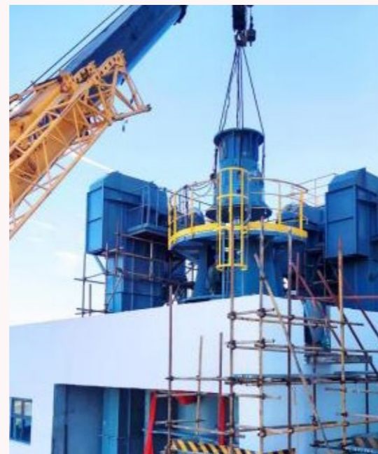
Successful installation of main equipment of the fly ash fine processing project at Jiaying Power Plant of Zhejiang Provincial Energy Group Company Ltd.
